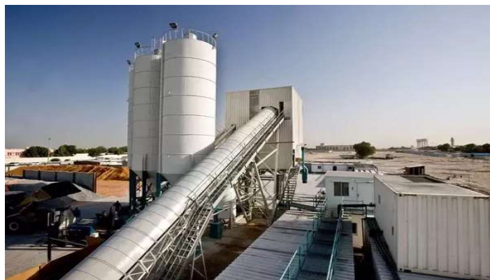
Figure 4.7: Batching Plant (Kabul, Afghanistan) operated by Firm B
