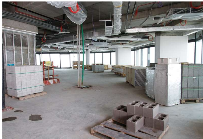
Figure 2.6: Examples of poor (up) and good (down) housekeeping in construction site
