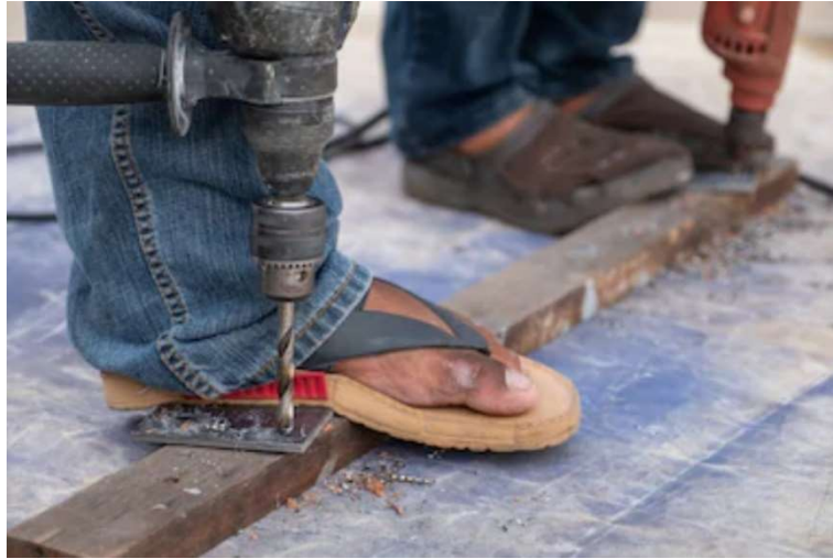
Figure 2.5: Example of improper footwear on the construction site
