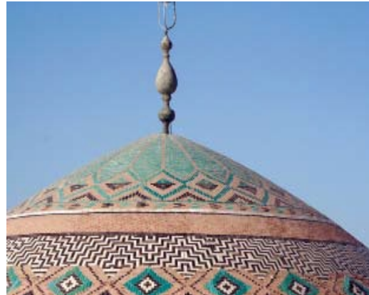
Figure 14: the broken lines, the top edge of the dome, Great Mosque
