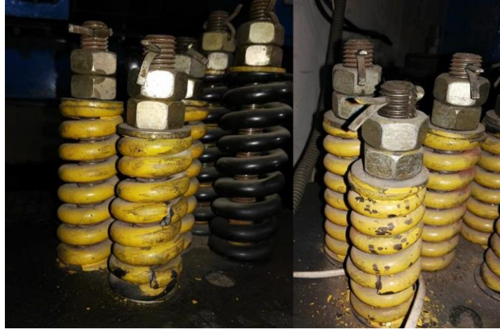
Figure 2.6: Broken springs of shackle rod in the elevator machine room
