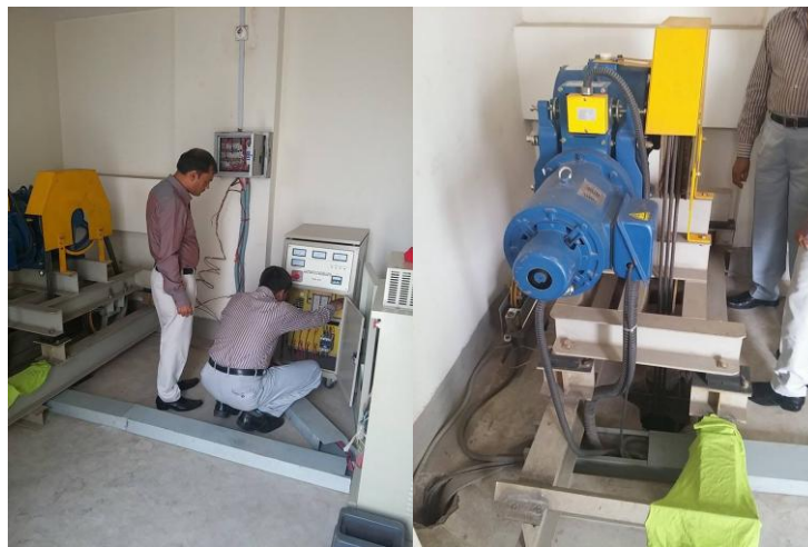
Figure 2.9: Elevator machine room – geared motor type with VVVF controller
