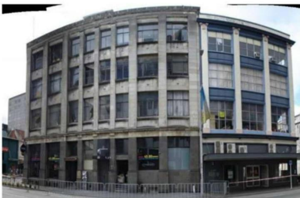
(a) Two four-floor damages due to pounding.
