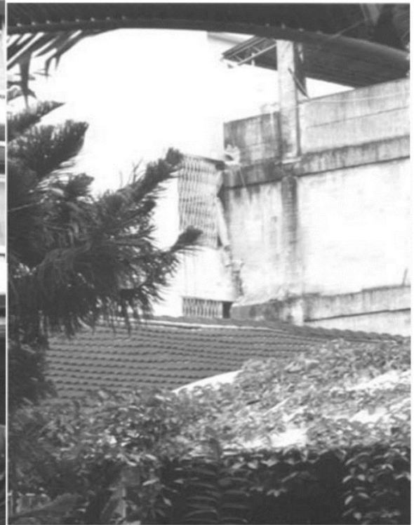
(c) Minor damage due to pounding
