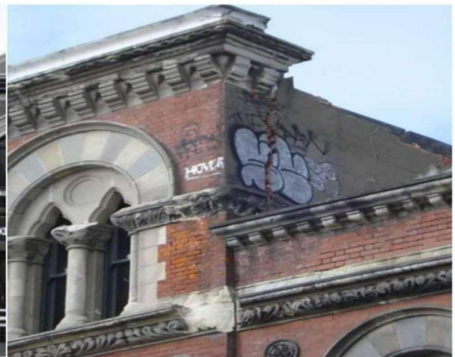
(b) Magnification of damage location(a).
