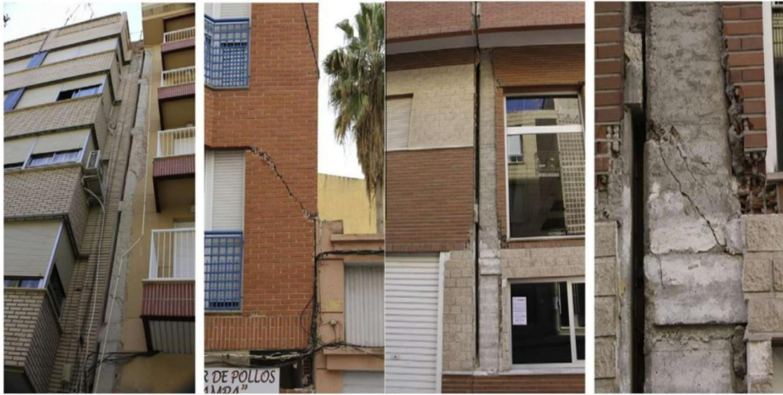
(a) Masonry damage due to the pounding.
