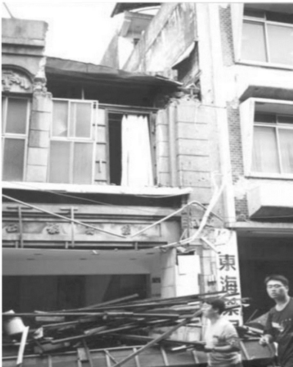
(b) Major damage due to pounding
