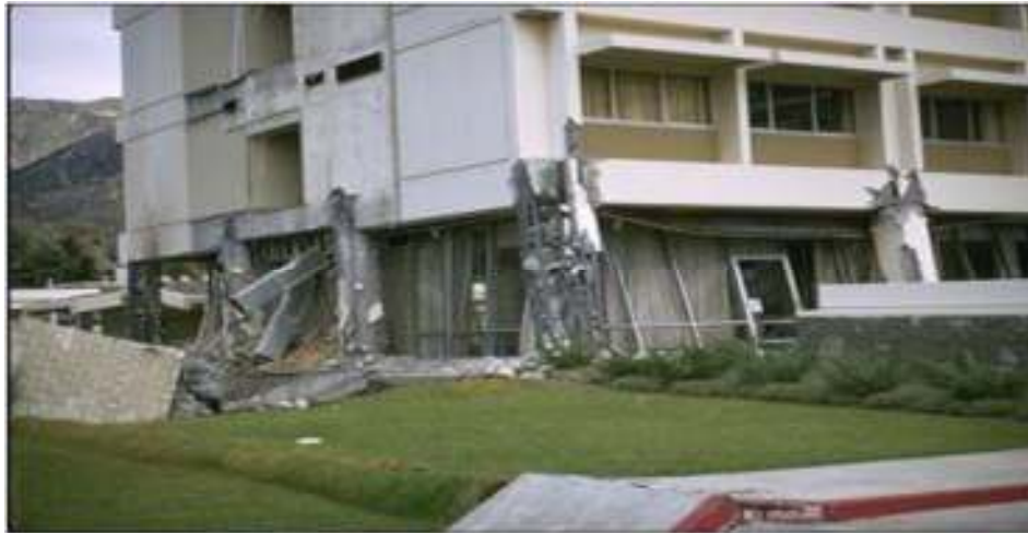
Figure 1.6: Failure of Olive View Medical State Center
