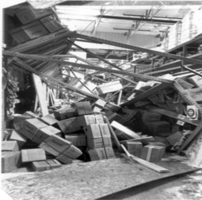
Figure 7: Collapse of a rack structure at the Santa Clarita Store [2]
