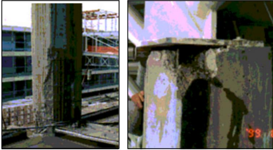
Figure 1.1: Observed Damage to the Terminal Building; base of third story column (left) and base of roof truss connection to column (right). (Constantinou et al, 1999)
